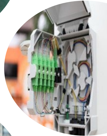
Fiber or splice degradation
